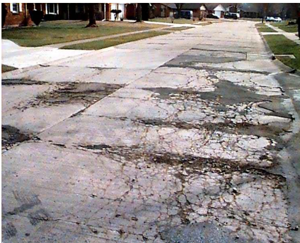
CONCRETE STREET DETERIORATION PRIOR TO PASSAGE OF STREET LEVY
