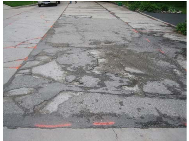
DETERIORATED CONCRETE WITH FAILING ASPHALT PATCHING
