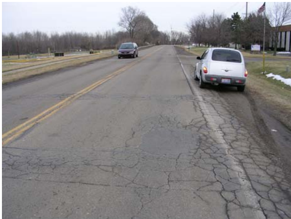
DETERIORATED ASPHALT PAVEMENT ON YELLOW SPRINGS-FAIRFIELD ROAD.
